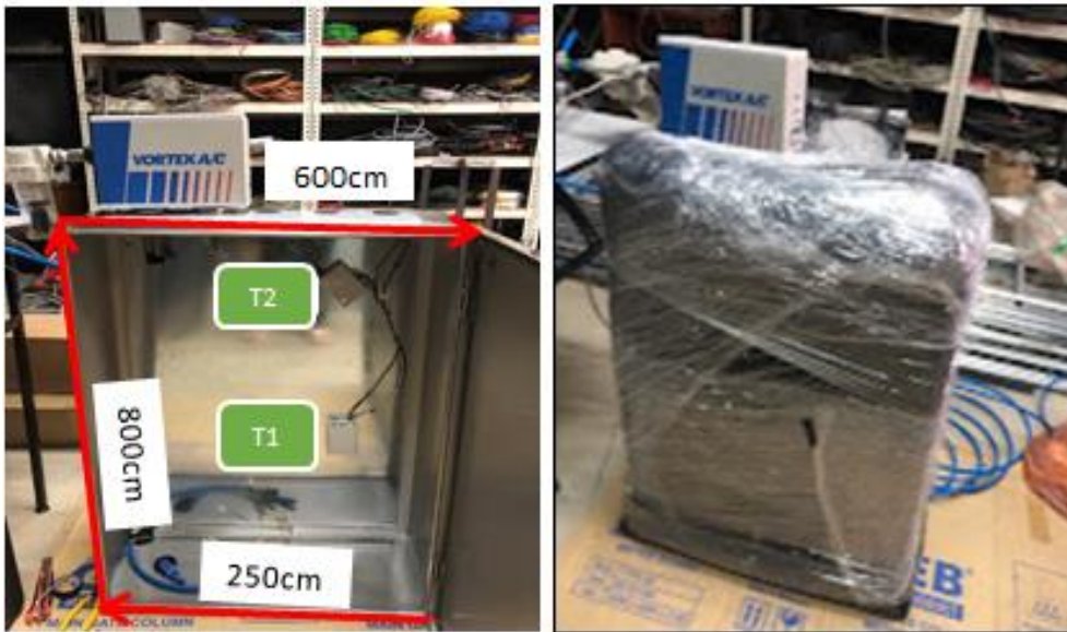
Figure 2: The condition of the enclosure and the location of the sensors T1(outlet vortex) & T2(Enclosure)
